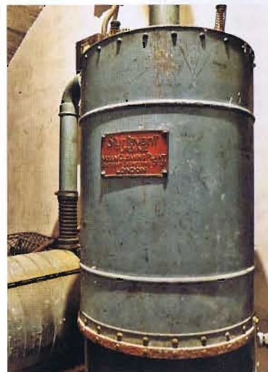
The central vacuum plant in the basement
