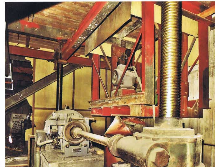
Conductor's lift carried within the central orchestra pit elevator
